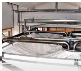
Loading and venting piping
